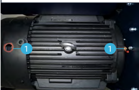
Motor for pump—grease points (1)
